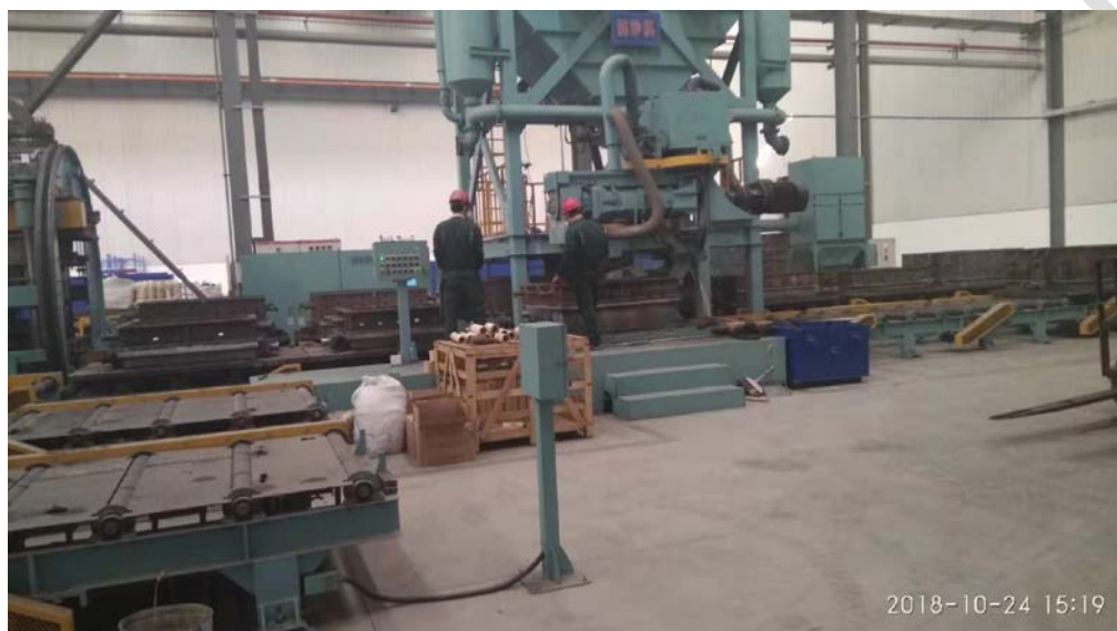
Figure 4 Alkaline phenolic resin bonded Kailin Ceramic Foundry Sand molding line in Shandong Province (P.S.: Due to the technical confidentiality of the company, specific technical parameters cannot be provided)
